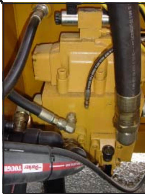
Figure 7-E. Drive Manifold Installed
